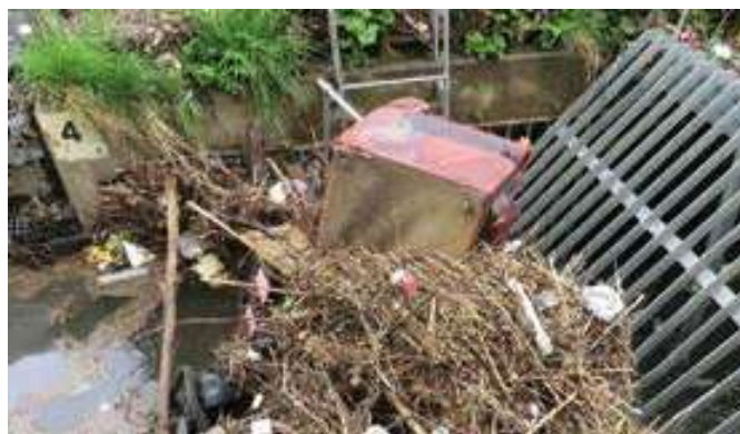
locked up culvert
