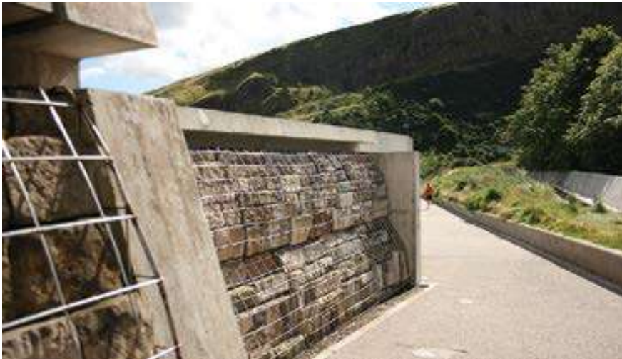
Reusing building materials—Holyrood Road Stone from the partially demolished Queensberry House was used in the walls on the exterior of the Scottish Parliament.
