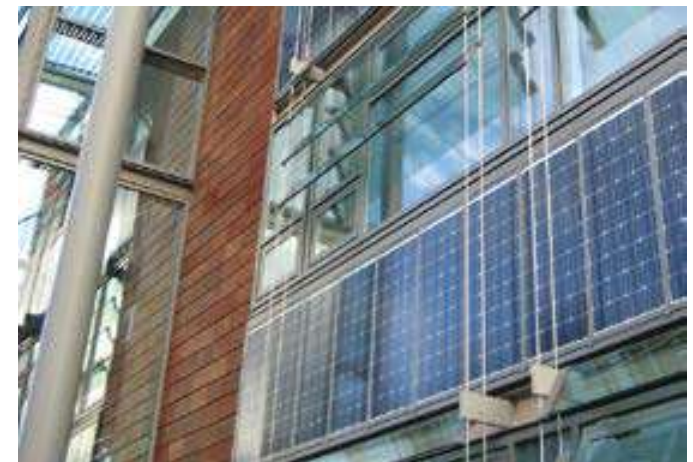
Integrating micro renewables—Kings Buildings Solar Panels are integrated into the design of the elevation.
